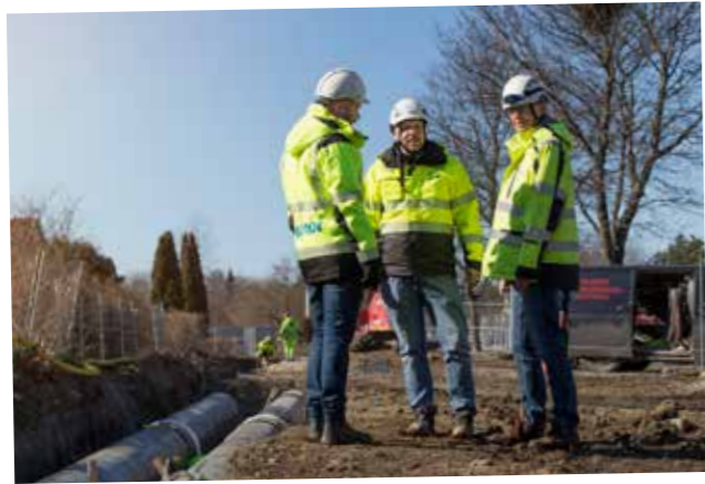
Tobias Thorell (left) of Uponor, Rikard Söderström of Fjärrvärmeprojekt Sverige AB and Hans Jakobsson of Stockholm Exergi visited the site at the early stage of the project.
